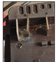
Ill. 1. Verdigris build-up
